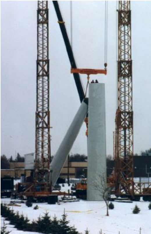
Placement of wind turbine tower sections Photo Courtesy of D. Pierson, Forest City, IA
