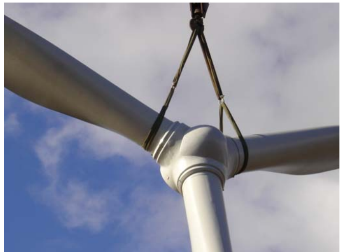
Photo of a crane lifting a three blade rotor hub up to nacelle for mounting to the generator drive.
