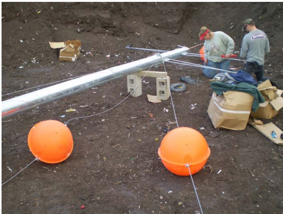
Top end of a typical 50m sectional tower
